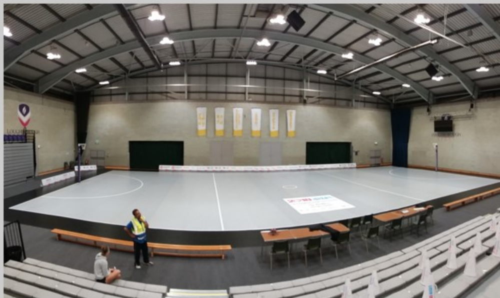
Foam backed vinyl layer installed over sprung timber surface at Loughborough University
